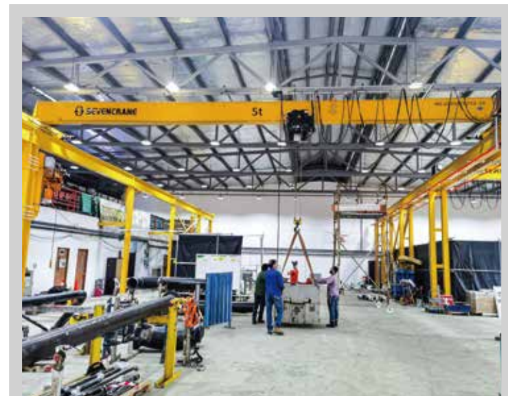
Vacuum Spreader Paper Roll Crane
