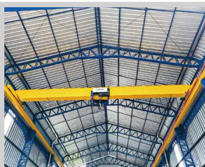
Handling Bridge Crane In Paper Workshop
