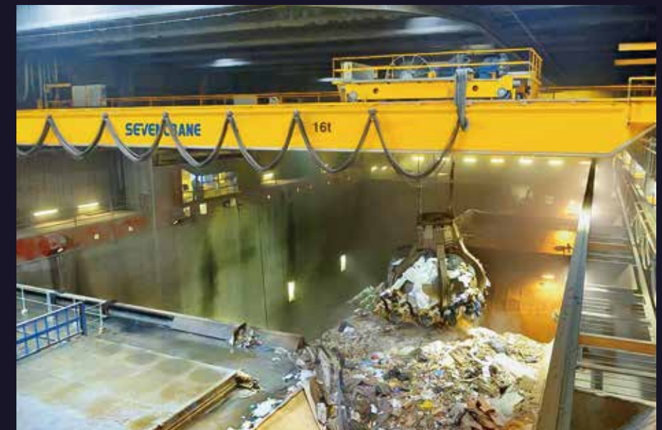
Fully Automatic Garbage Handling Traveling Crane
